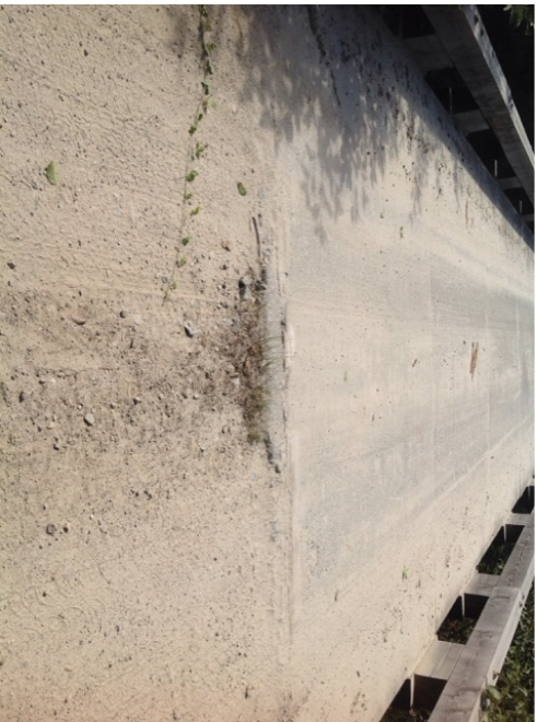
left ballast wall at road surface damage
